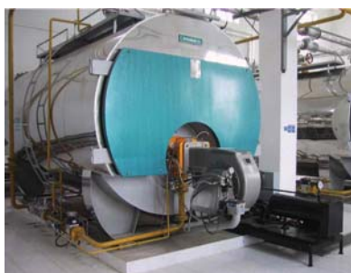
Figure 4b Small boiler.
